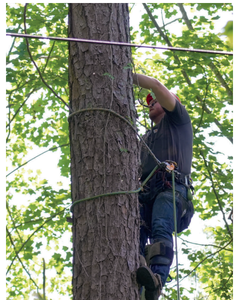
BREC Tree Specialist Ethan Jordan works in a heavily wooded area to clear a tree growing near a power line.
