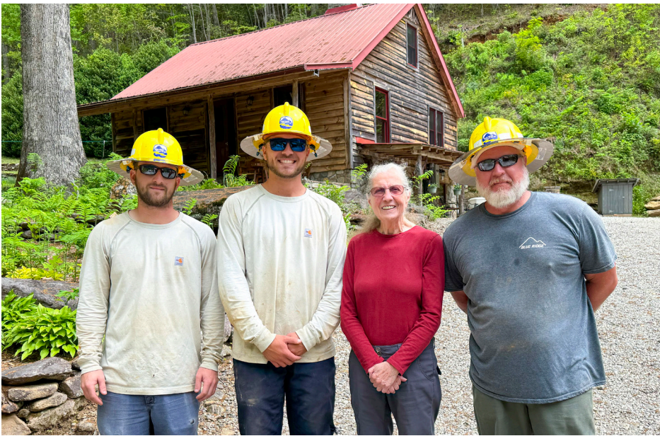
A BREC crew visits with member Marnie Sutton after changing out a pole near her home in Rocky Bottom that had been clawed by bears and tilted by Hurricane Helene. Sutton's home is the last meter on our system before you enter North Carolina from Pickens County. Pictured are (left to right linemen) Zeke Thompson and Grayson Pace, Sutton and Line Foreman Anson Perry.
