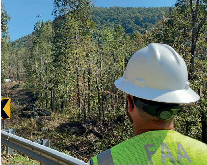
A drone was used to pull wire across areas that were inaccessible by truck. Without these “mobile linemen,” recovery time would have been longer.
