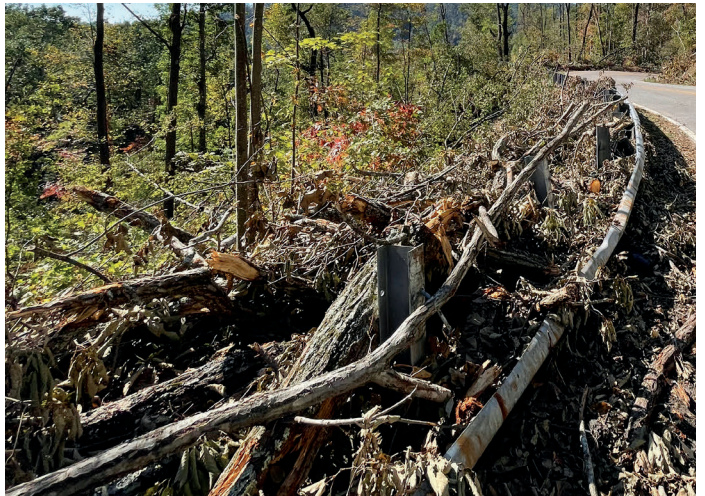
Helene’s high winds caused devastating damage along the scenic roads in the Rocky Bottom area, making travel dangerous for emergency vehicles and utility trucks.
